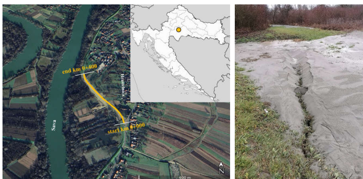
Figure 6. The layout of the damaged section of Hrastelnica levee with observed sand ejecta
