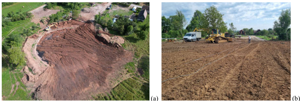
Figure 12. Installation of final layer of clay cap (a) and the terrain surface after the remediation works with SASW control quality work being conducted (right)
