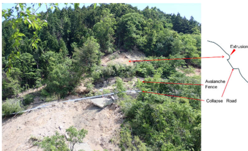
Figure 13. Image and Simplified sketch (cross-section) at Loc. VII. Extruded area at the southern end of the landslide
