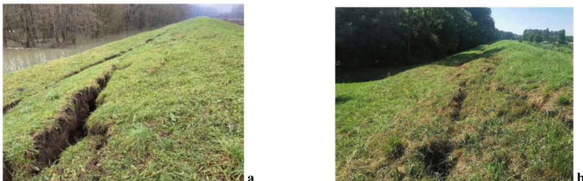
Figure 1. Comparison of the levee crack: a) immediately after the earthquake and b) after 6 months
