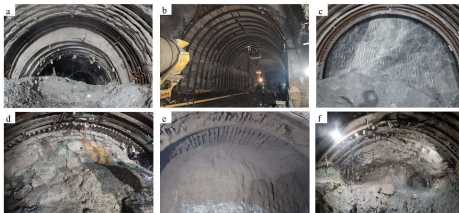
Figure 5. Showing Photographs of rectification works and additional support measures (a) restoration work under progress, skin to skin ribs were embedded under SFRS (b) Rectified tunnel (c) Fore poling to stabilise the crown of the Tunnel. (d) & (e) Pipe roofing created an umbrella-like structure above the crown to prevent collapses. (f) Multisegmental excavation.
